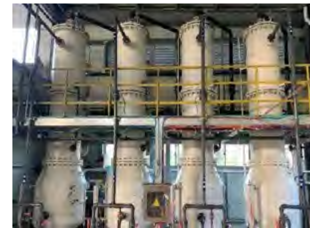
Helium gas recovery equipment
